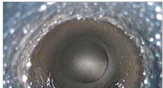
Supply tube view from the locating flange area towards the elbow transition
